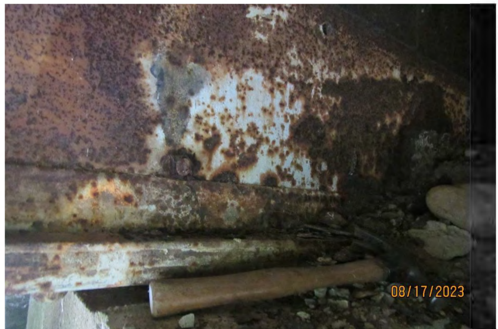
Photo 10 – Corrosion in east girder end at 5 th bearing from north side
