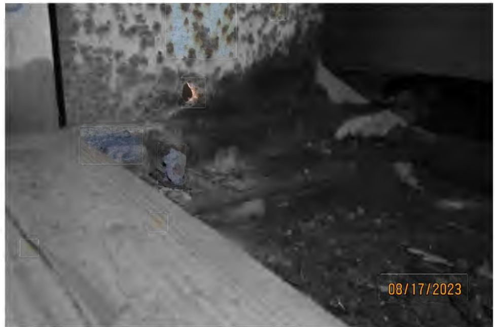
Photo 9 – Corrosion in east girder end at 2 nd bearing from north side
