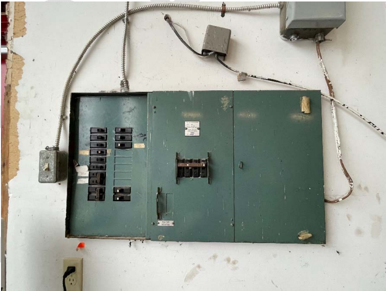
Figure 10 – Main Electrical Panel
