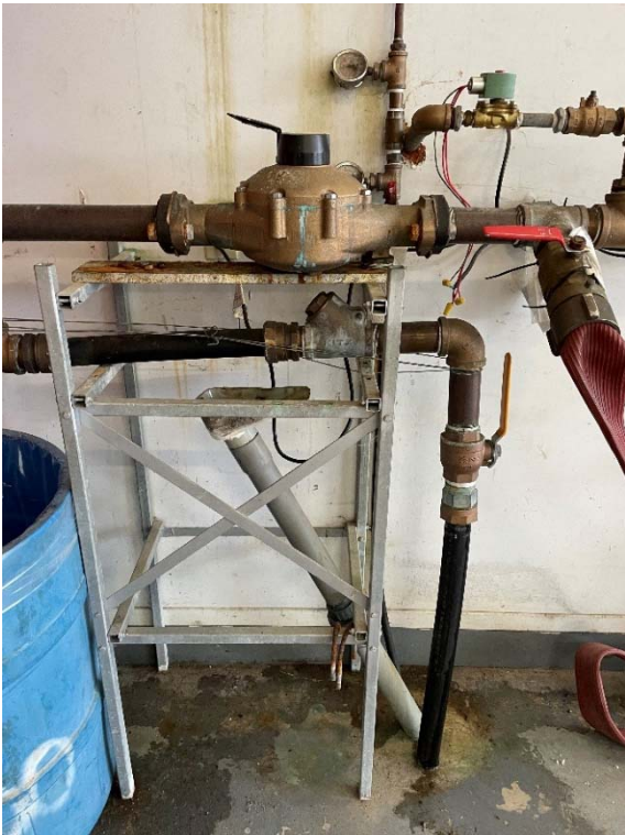
Figure 13 – Water Distribution Equipment
