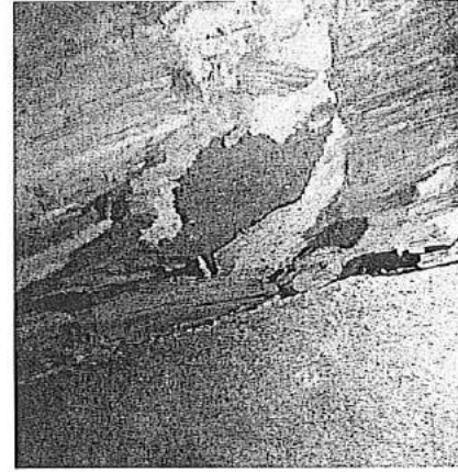
Photograph 4 Water damaged floor boards and paper supporting confirmed mould growth below the east portion of the office.
